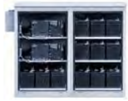
Dual PN-3 2 Power Supplies 4 Battery Strings
