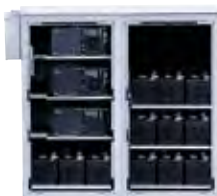
Dual PN-4 3 Power Supplies 4 Battery Strings
