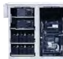
PN-4/CE-9X2 2 Power Supplies 3 Battery String AlphaGen™ Generator
