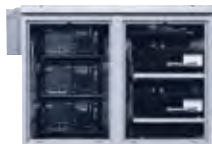
PN-6 3 Power Modules 2 48V Battery strings
