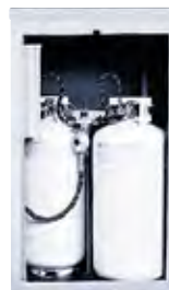
CE-3/9G Propane Storage for Generator
